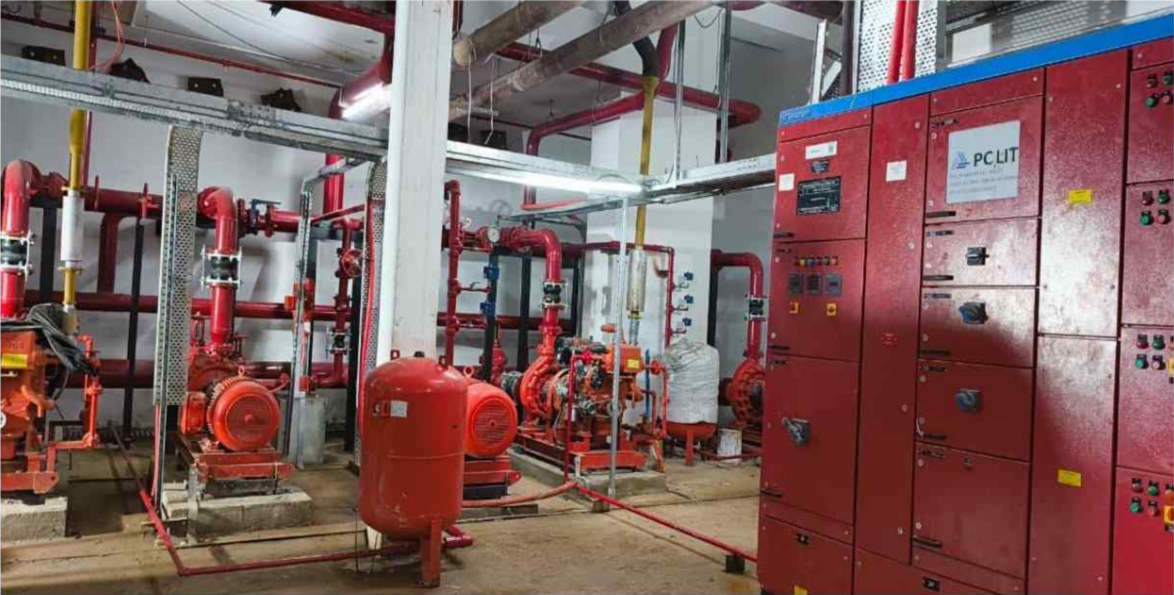
Photograph of fire-fighting systems
